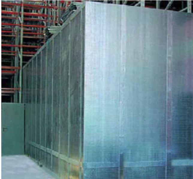
An Acoustic Enclosure.
