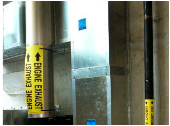
A fire-rated pipe enclosure.
