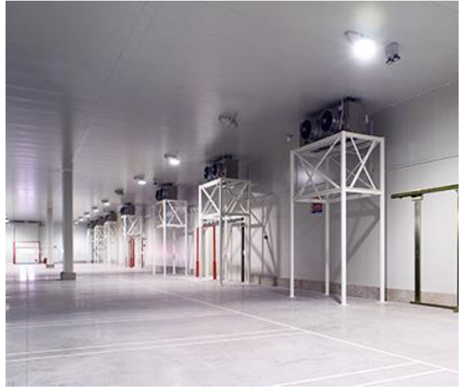
DuraWall™ utilized in a climate controlled facility.
