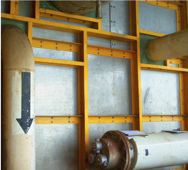
H0 wall with pipe penetration seals.
