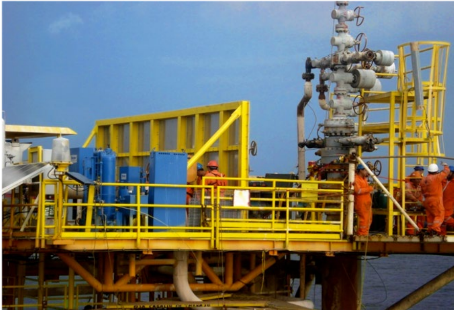
A DuraBlast Barrier protecting control panels.
