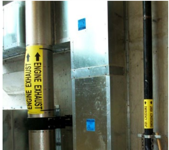
A fire-rated pipe enclosure.
