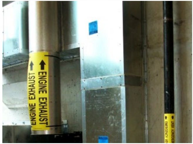
A fire-rated pipe enclosure.
