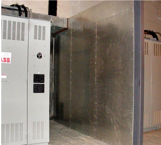
A fire wall separating two electrical enclosures.
