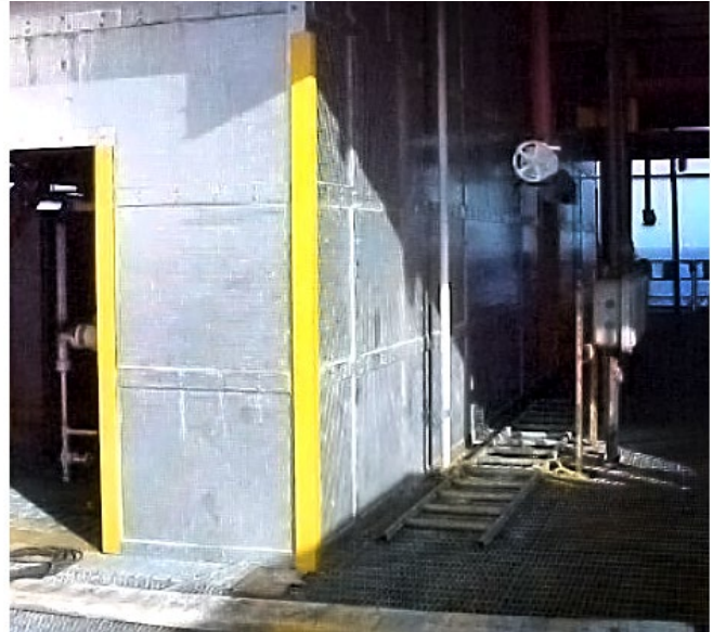
H120 wall protecting equipment.
