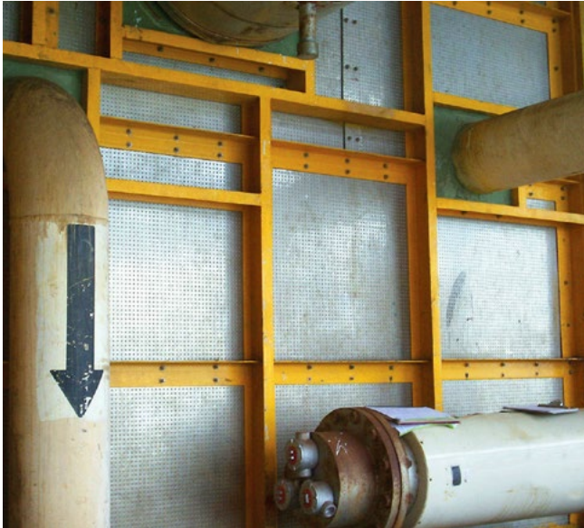
H0 wall with pipe penetration seals.
